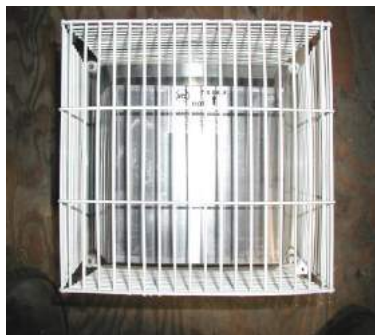
VIEW OF SAFETY CAGE
